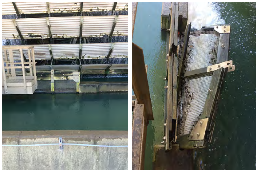
Figure 3. Cooling tower fill collapse (left), broken screens and debris (right).
